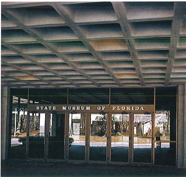
Figure 23-10. Waffle construction is used in this structure to form the roof slab. Spans of up to 60' are possible.
