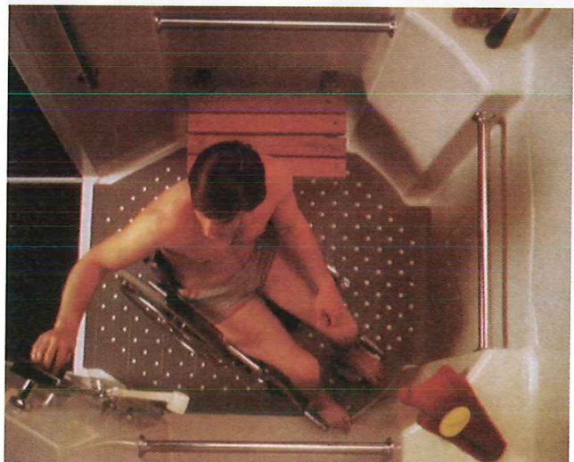
Figure 7-32. The floor area of the shower unit permits a 5' turning radius for wheelchairs. Several grab bars are within easy reach. (Universal-Rundle Corporation)
