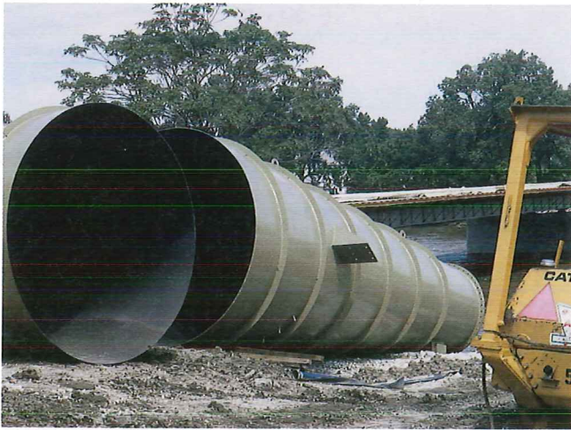
Figure 17-17. These large steel intake tubes for a hydroelectric generating plant were fabricated as a subassembly in the shop and shipped to the job site.
