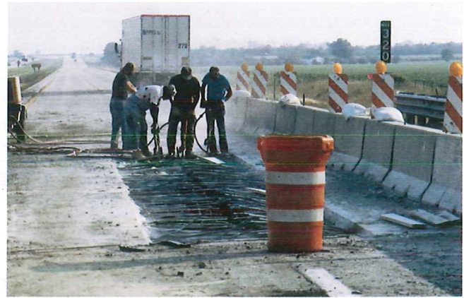
Figure 17-19. Steel reinforcing rods, like those exposed here during a bridge deck repair project, are embedded in concrete to provide strength. In addition to paving use, reinforced concrete is widely used for structures. (Jack Klasey)
